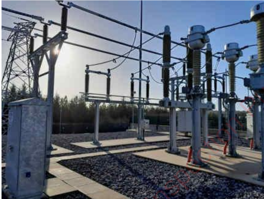
Plate 2-3 Typical 110kV electrical infrastructure
