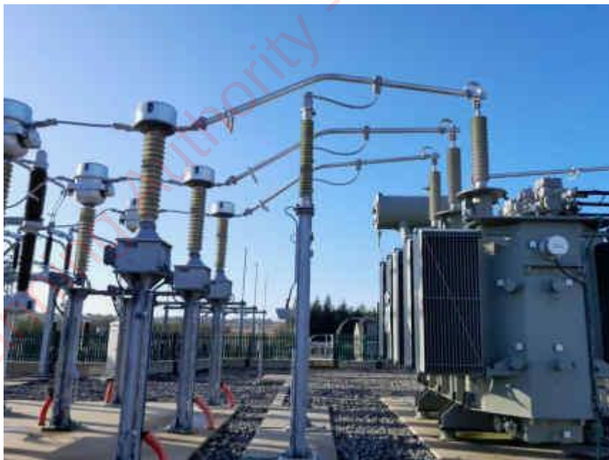
Plate 2-4 Typical 110kV transformer connection
