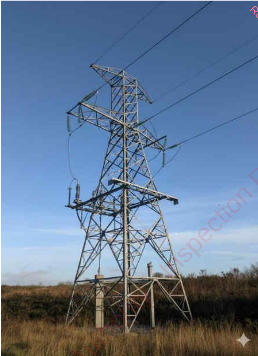
Plate 2-12 Cable end mast
